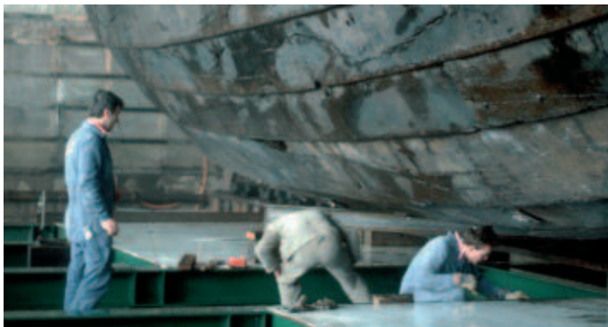
Fig. 5 - Building the stainless-steel conservation tank around the reconstructed cog (Photo: P. Hoffmann, DSM)
